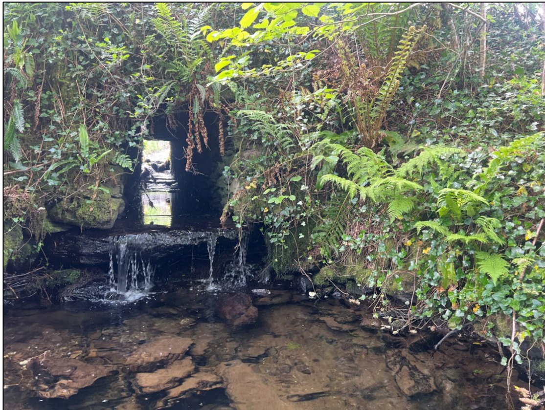
Plate 4-34. A representative picture of the under-road box culvert and raised apron at the upstream survey extent of GC 8.
