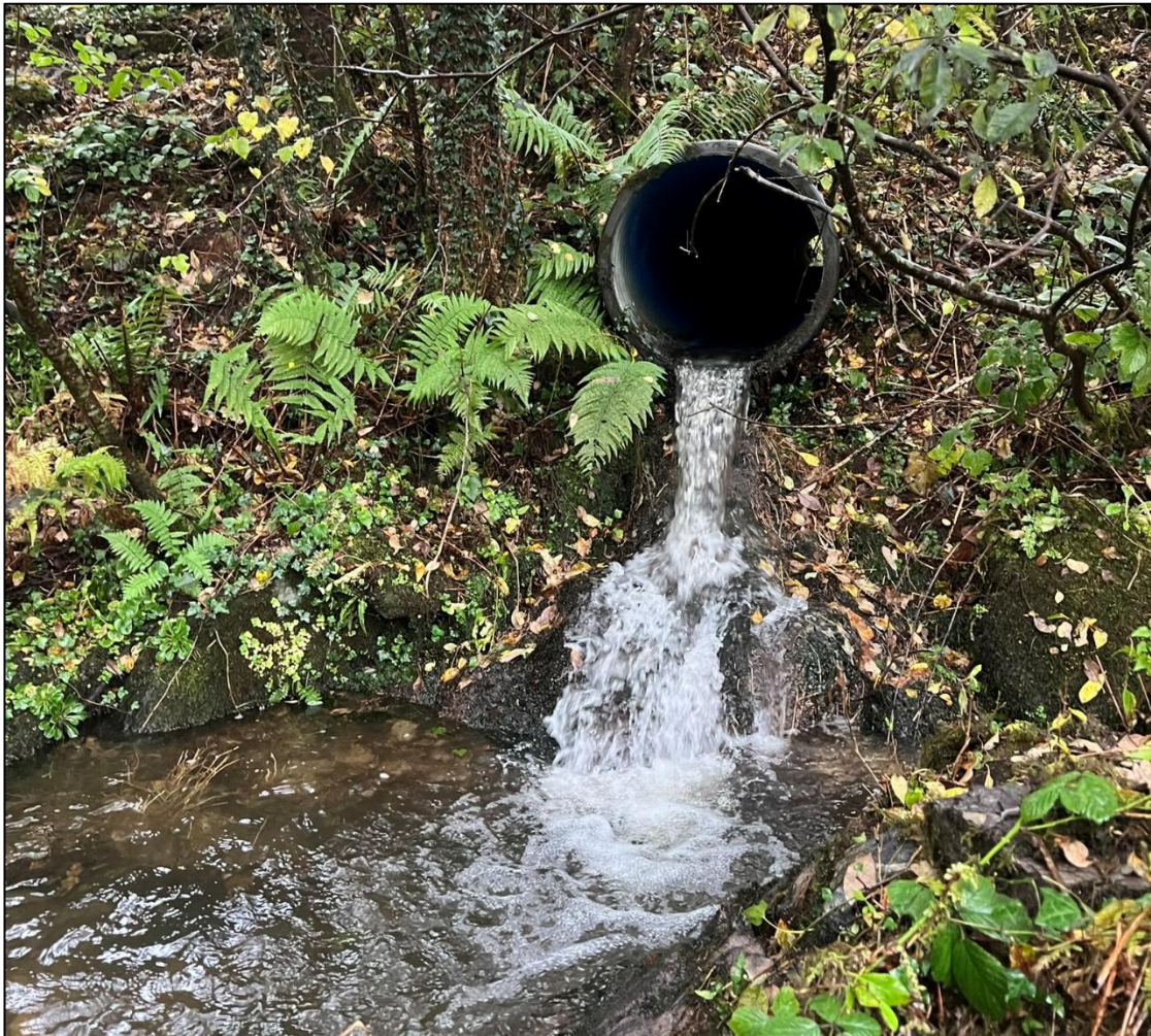
Plate 4-29. A representative picture of the pipe culvert at the upstream survey extent of GC 4
